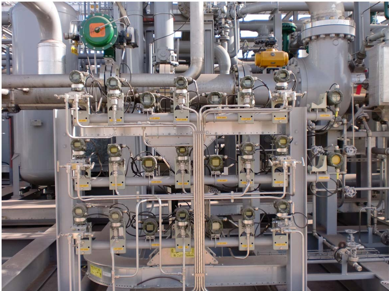
Figure 11: Remote mounted instrumentation racks allow operations staff to easily view the device from the skid edge.
