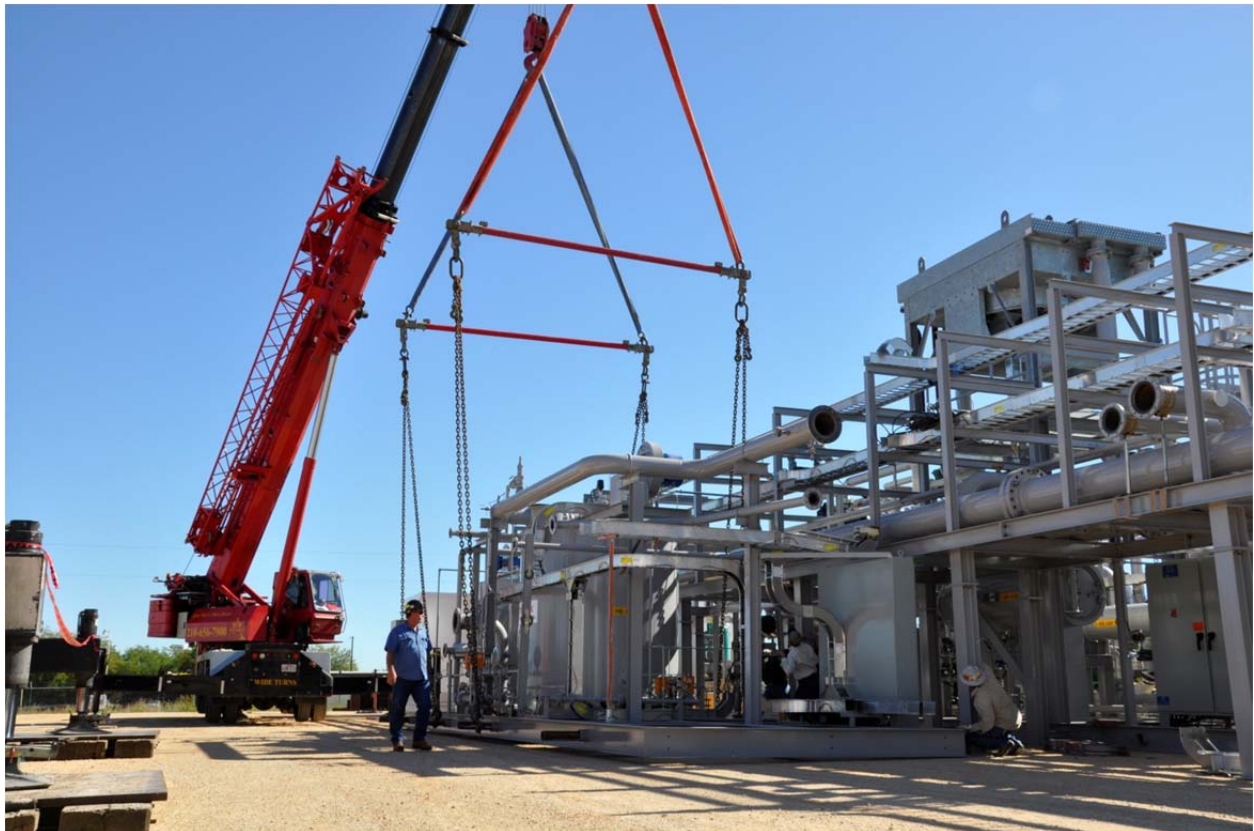
Figure 21: Piping aligned during the setup process
