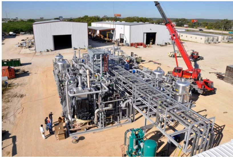
Figure 22: Final set up of the process modules and interconnecting cable tray to the control building
