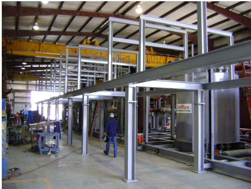
Figure 7: Multiple process modules are set up in the manufacturing space before piping begins.
