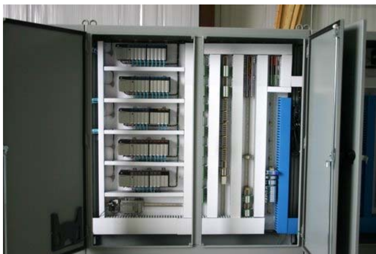
Figure 10: Main PLC control panel.
