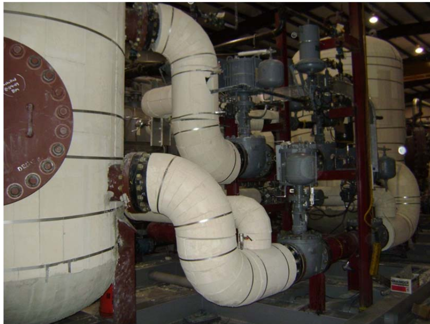
Figure 9: Calcium silicate block insulation is installed on vessels. Preformed piping insulation is miter cut to create custom fit.
