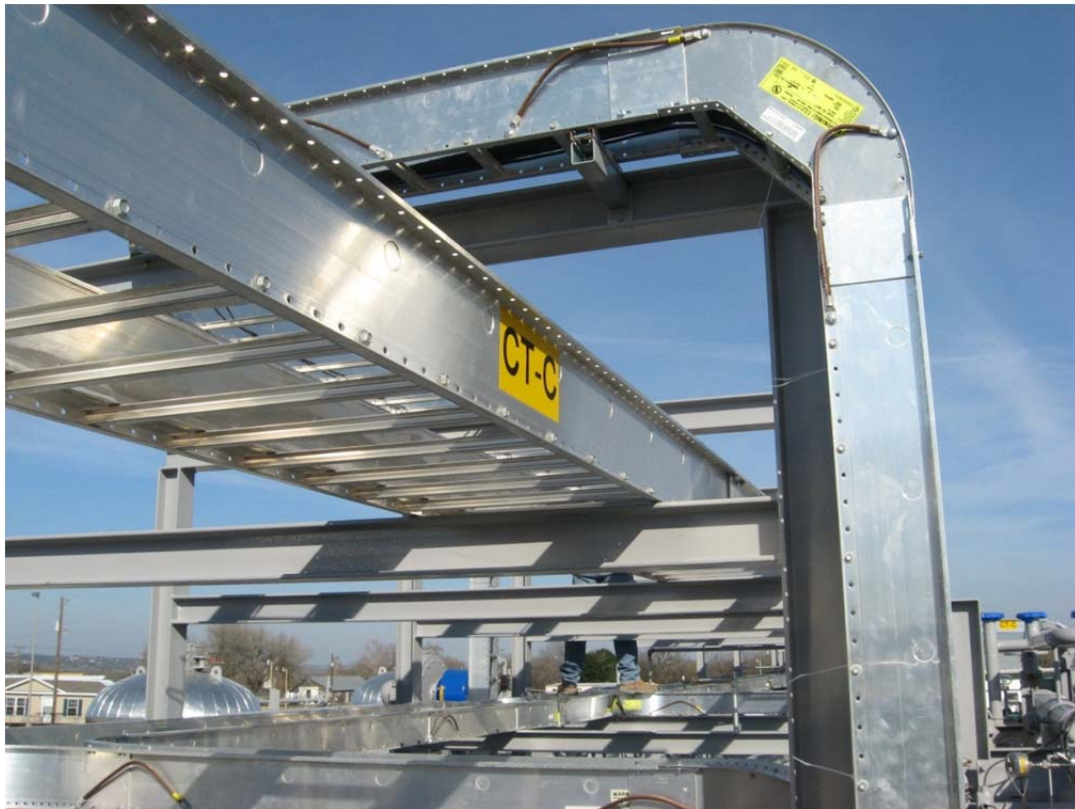
Figure 14: A labyrinth of cable tray keeps the installation clean and the plant running smooth.
