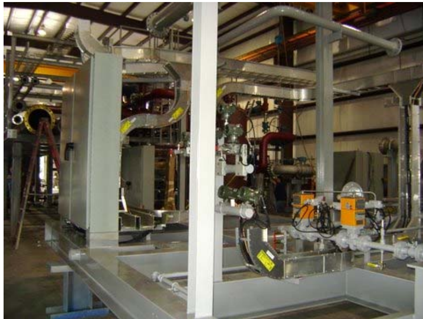
Figure 12: Module cable tray and wiring from panel to device.
