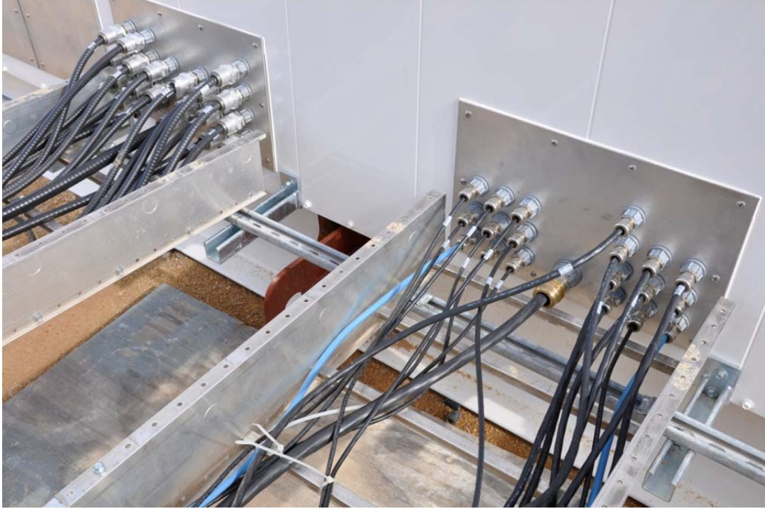
Figure 13: Field wiring connections are test fit to the control buildings to increase quality and efficiency.
