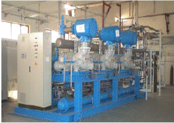
Helium Screw Compressors Station
